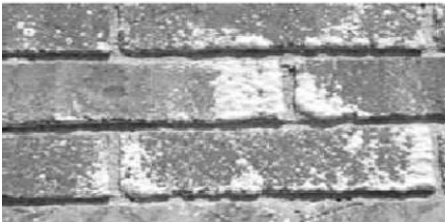
Figure.1 Brick Masonry wall subjected to efflorescence [10]
